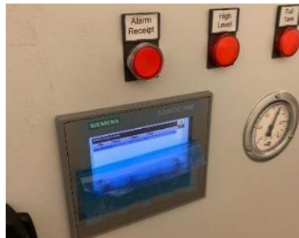
System Control Panel
