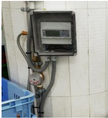
Electric & Water Meter
